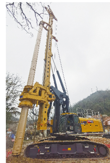
XR460E助力贵阳融创国宾道城市综合体项目施工 XR460E helps the construction of Guiyang rongchuang Guobindao urban complex project
