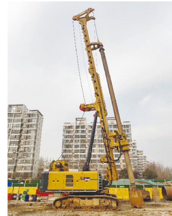
10台徐工旋挖钻机助力徐州南三环施工 10 sets of XCMG rotary drilling rigs assist the construction of South Third Ring Road in Xuzhou
