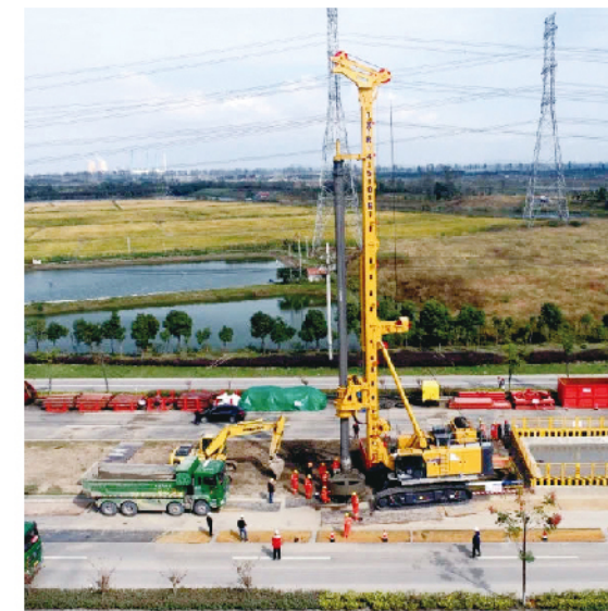
XR450E在浙江绍兴杭绍甬高速复线项目施工 XR450E works in Hangzhou Shaoxing Ningbo Expressway double track project in Shaoxing, Zhejiang Province
