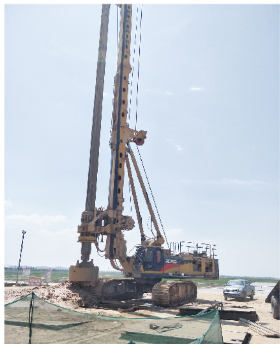
XR460D旋挖钻在银川石嘴山黄河大桥施工 XR460D rotary drilling rig works for the construction of Shizuishan Yellow River Bridge in Yinchuan
