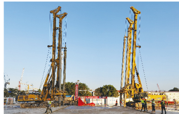
徐工旋挖钻机助力深圳南山联合科技大厦 XCMG rotary drilling rigs help the construction of Shenzhen Nanshan United Technology Building
