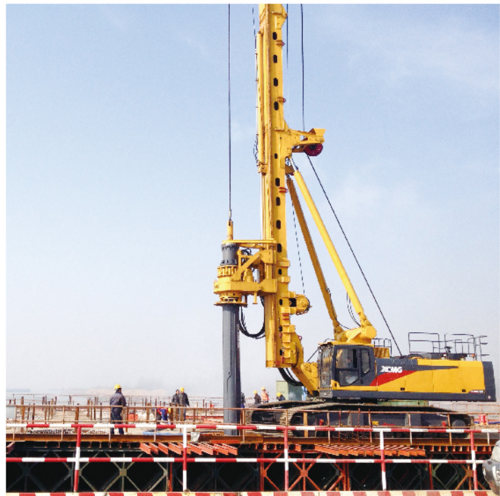
徐工XR460D旋挖钻机在安徽芜湖进行芜湖大桥项目施工 XCMG XR460D rotary drilling rig works for the construction of Wuhu bridge project in Wuhu, Anhui Province
