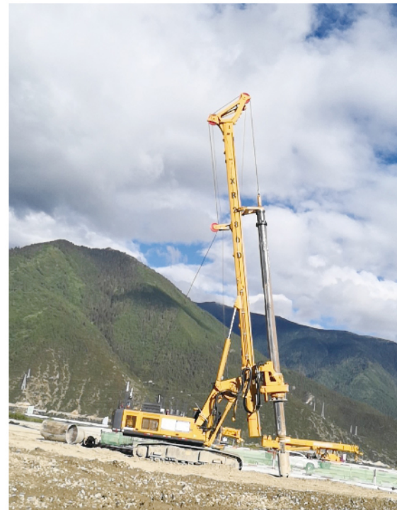
XR280D川藏铁路林芝火车站施工XR280D works in the onstruction of Linzhi railway station of Sichuan Tibet railway
