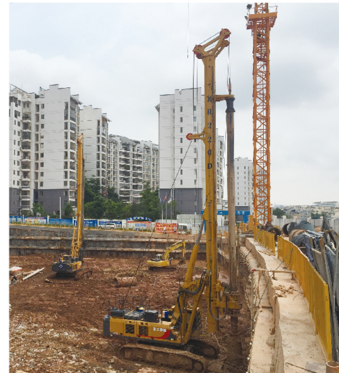
XR400E和XR200D在华夏基础柳州碧桂园十里江湾施工 XR400E and XR200D work in Shilijiangwan of Liuzhou Country Garden in Huaxia foundation
