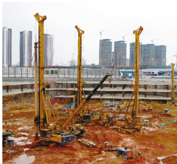
徐工XR120E旋挖钻机在河北雄安进行雄安高铁站项目施工 XCMG XR120E rotary drilling rigs carry out construction of Xiong'an high speed railway station project in Xiong'an, Hebei Province
