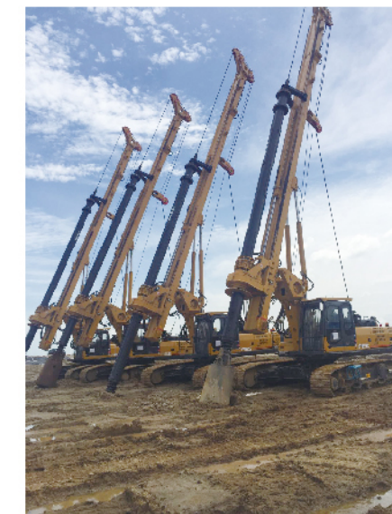
XR150DIII机群印尼万丹火电厂施工 A group of XR150DIII rotary drilling rigs work in the construction of Indonesia Wandan thermal power plant
