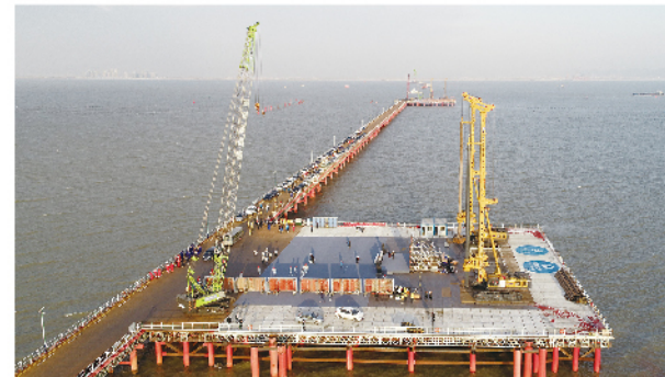
12台徐工旋挖钻机助力广东黄茅海跨海通道12 XCMG rotary drilling rigs work for the construction of Huangmao sea crossing channel in Guangdong
