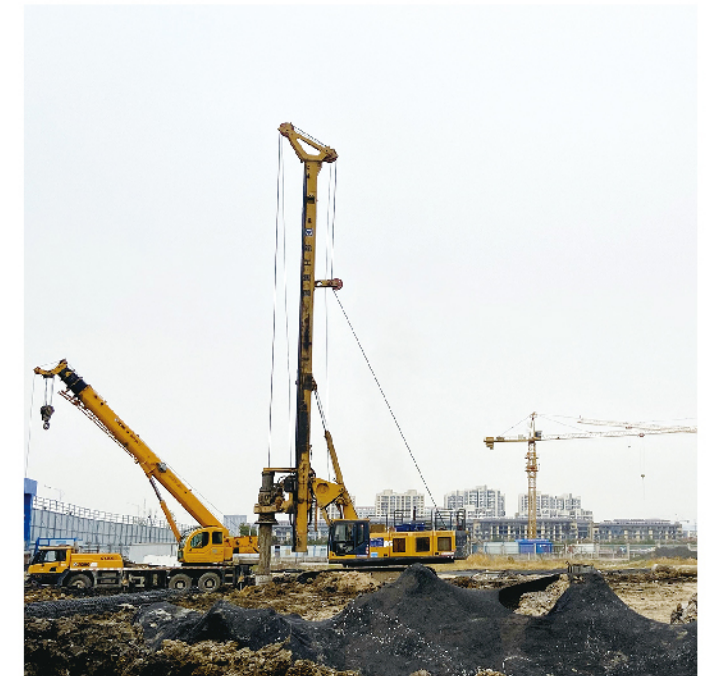
XR280E在徐州房建项目施工 XR280E works in Xuzhou housing construction project
