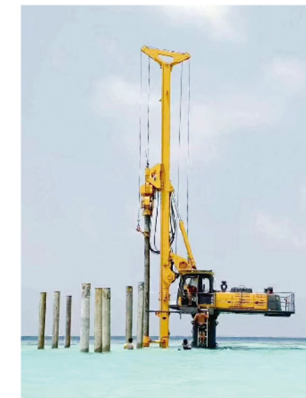
徐工XR160E在马尔代夫跨海大桥项目施工 XCMG XR160E works in the construction of sea crossing bridge in Maldives
